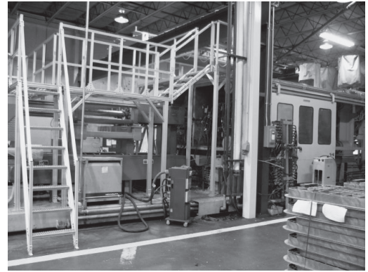
Moulding Press Catwalk
