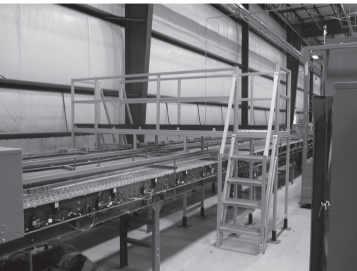
Large Conveyor Crossover
