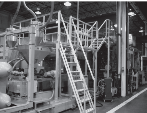
Custom Stairs and Platforms
